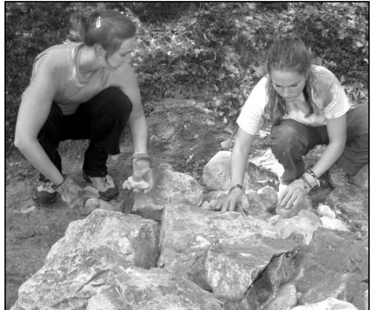
On a heavily eroded section of the Wildcat Notch Trail, these FBH volunteers helped create a tight base layer of rock that was carefully filled and covered with gravel and dirt. photo by Dexter Robinson
