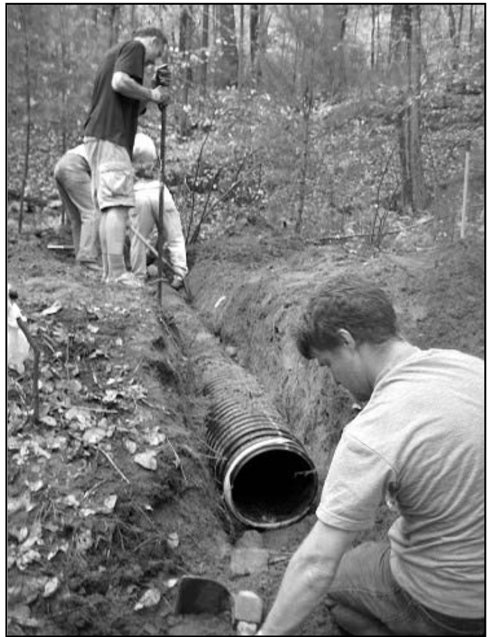
The Friends of the Blue Hills crew working on a typical Blue Hills culvert replacement project along Border Path. Photo by Dexter Robinson
